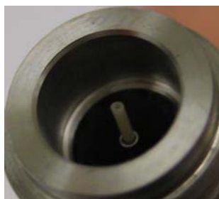
Sample line installed incorrectly
