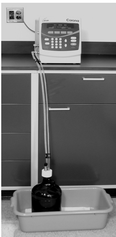
Figure E-11: Correct Setup of Drain Tubing (Note Secondary Containment)
